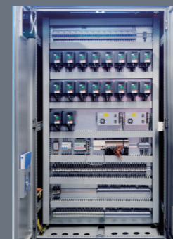
电柜 Electric cabinet
